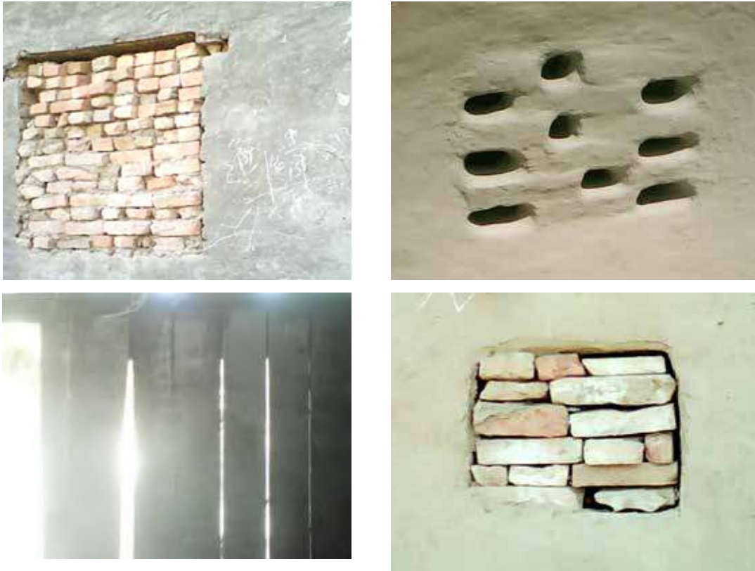
Figure 19 - Modifications made to windows by homeowners seeking to address concerns over privacy and security
