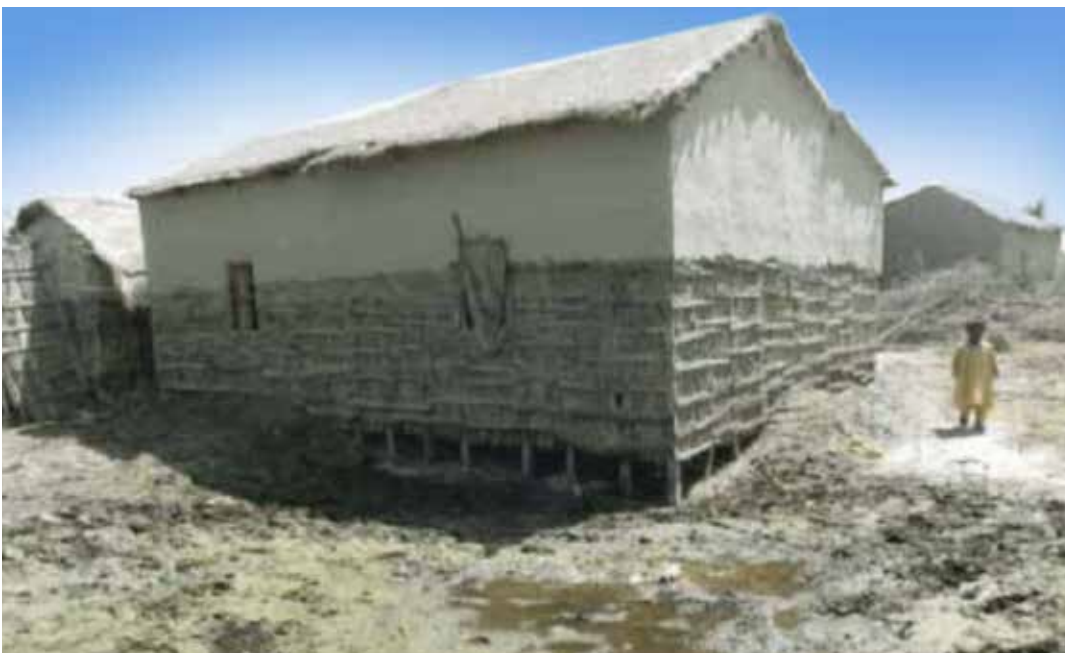
Figure 16 - Loh-kat shelter after flooding (UN-HABITAT 2010)
