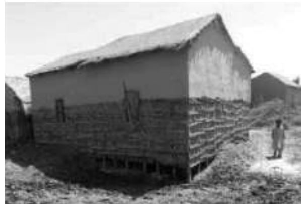
Figure 15: Example of flood damage to loh kat shelter
