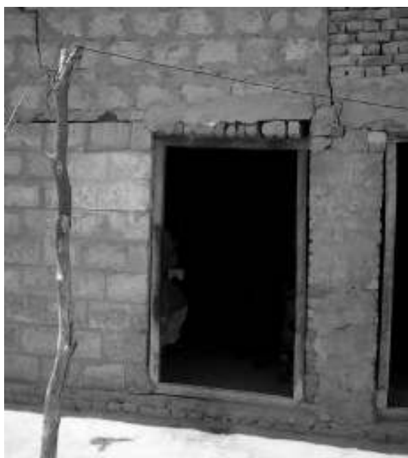
Figure 08: Example of low strength wall
